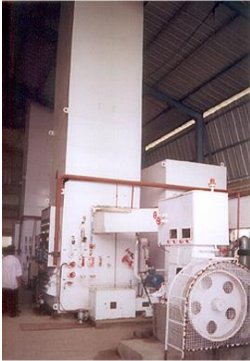
ASU & Expansion Engine of Oxygen Plant
