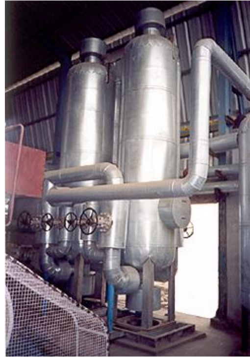
M.S. Battery for Oxygen Plant
